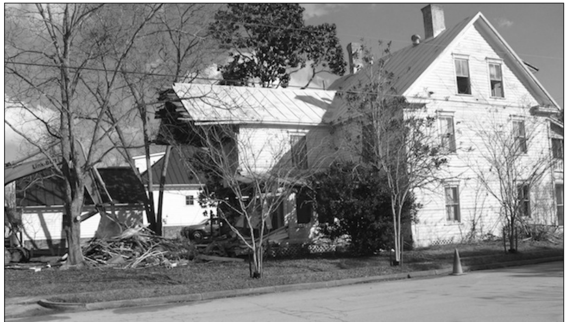
The Hinman House in Oriental, formally known as the Midyette House, was demolished last week. The home, at the corner of South & Wall Streets, dates back to the late 1800s and is among the oldest in town. At one time the home was host to an annual art class.
