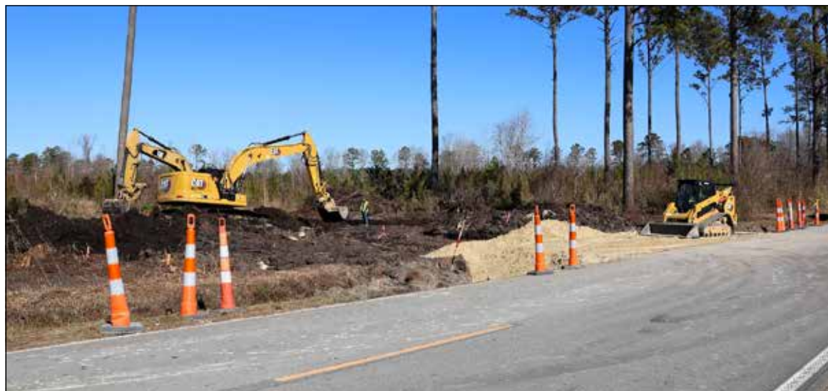
Driveway entrance construction off of Lee Landing Road and site clearing and prep are well underway.
