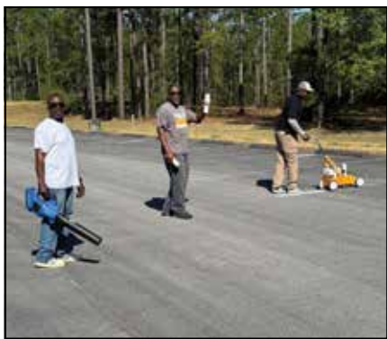
PCC Instructors Gregory Green, left, Maurice Smith, center, and Demetris Collins work on restriping the Delamar Center parking lot. Contributed photo
